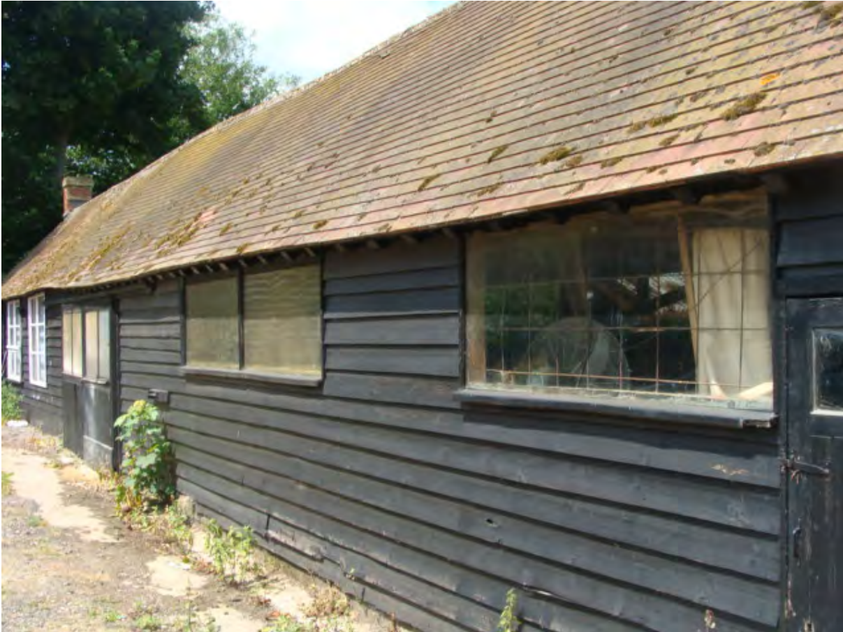
Picture 1.9 Curtilage listed storage building to south west of The Castle, worthy of retention.
